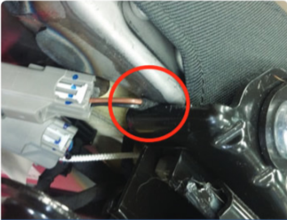
Fuel fill valve Heater element harnesses near the rear inboard corner of the seat assembly
