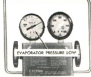
FIGURE 7—TXV STUCK CLOSED
