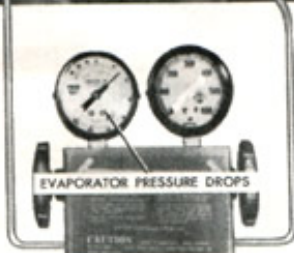
FIGURE 5—POA VALVE STUCK OPEN
